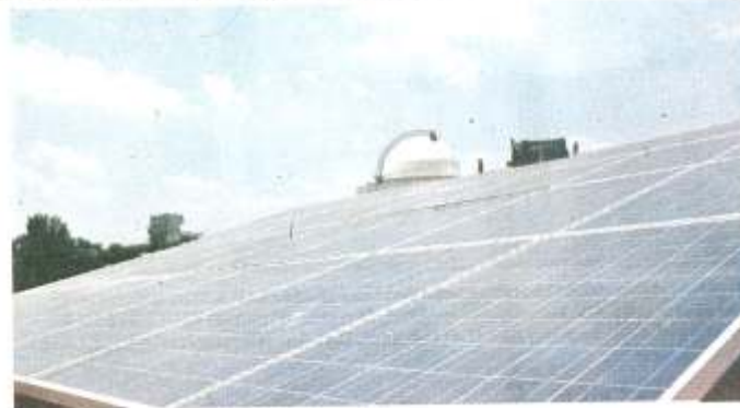
The solar panel in St Joseph's College of Arts and Science
